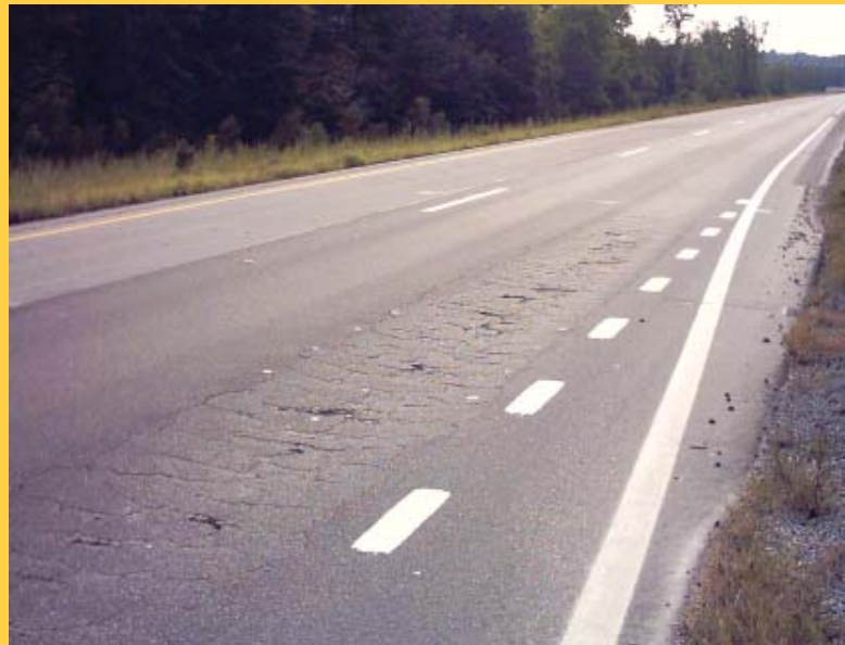
Photograph A. Fatigue cracking in Structural Test Section N1
