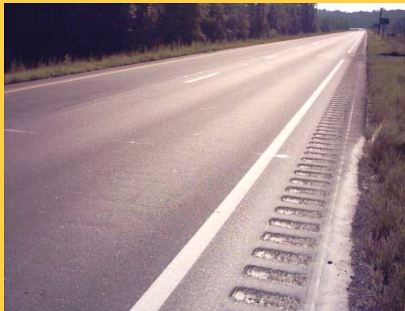
Photograph B. Fatigue cracking in Structural Test Section N2
